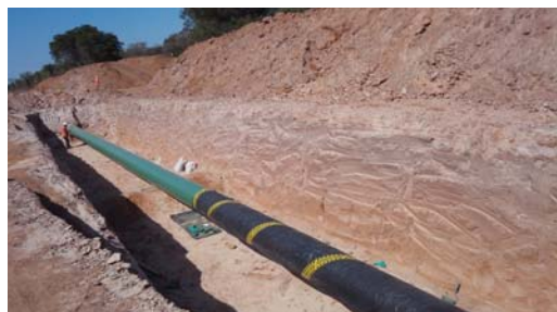
doing QC checking at the end of the day while protecting a sand blasted stretch.
