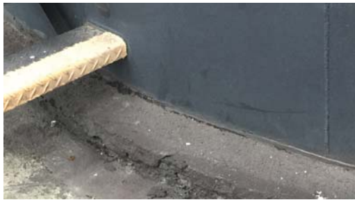
Tank bases showing signs of corrosion with cracked / crumbling concrete bases.
