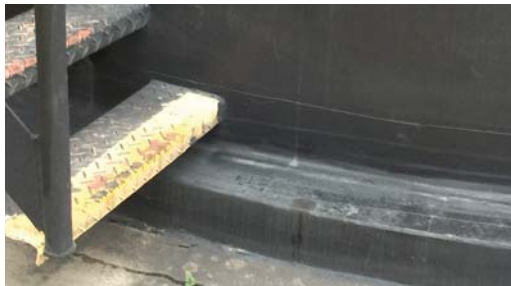
The same tank base now protected with Premier Coatings Tank Base Protection System.
