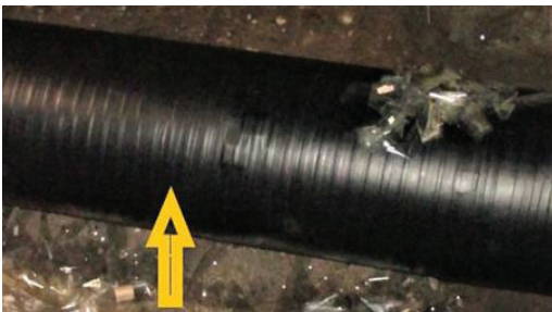
Pipe completed with Premcote Butyl 35 to provide corrosion prevention for years to come.
